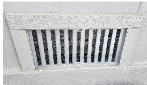
Proper operable crawl space vent that opens and closes
