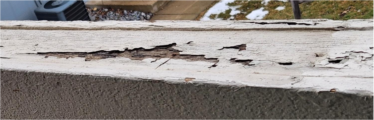
Original balcony railing top showing dished top which catches rain and promotes rot
