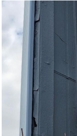
Trim board under downspout in bad shape – often an indicator that the old downspout split on the back and needs to be replaced
