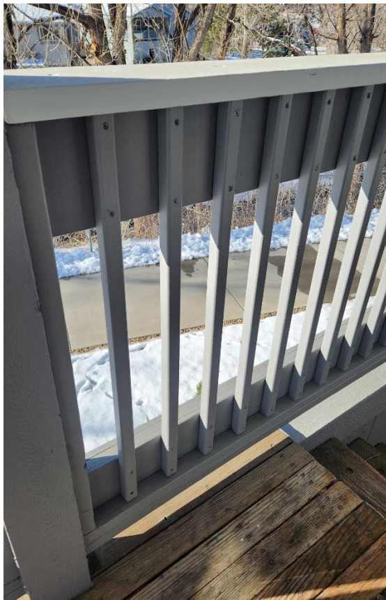
New railing design which meets code & deters wasps
