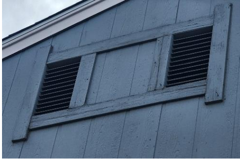
Attic vents with rotten trim
