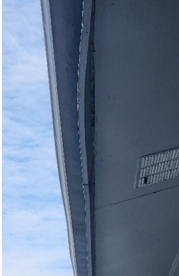
Bowed fascia board
