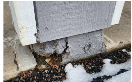
Crumbled concrete pier
