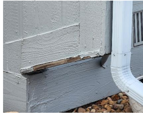
Wing wall deterioration
