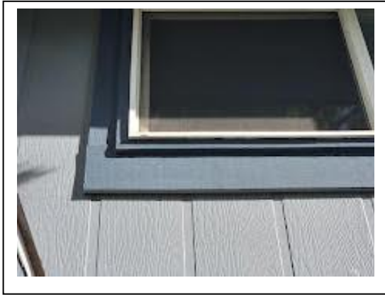
Trim not removed, window not inserted far enough into wall opening, so extra trim added.
