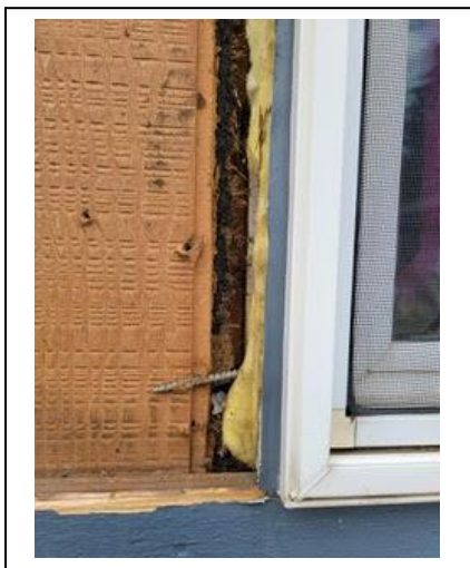
Screw between siding and trim
